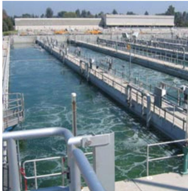
Phase I Aeration System Testing
